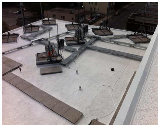
Communication Tower Roof
